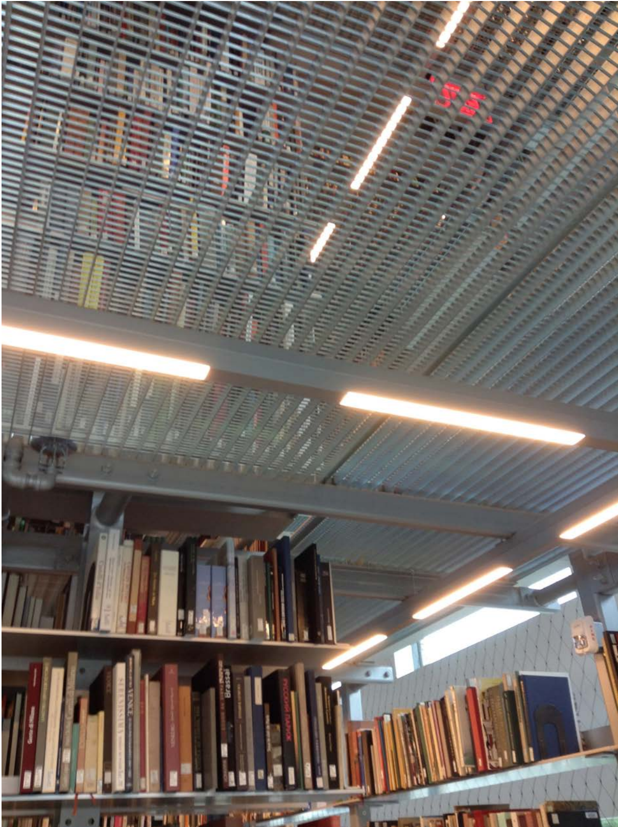
Figure 12. Perforated floor panels violate basic principles of compartmentation by connecting more than two stories; larger “6-inch flue” openings also appear in each story under the bookstacks. Photo by Jonathan Ochshorn.
